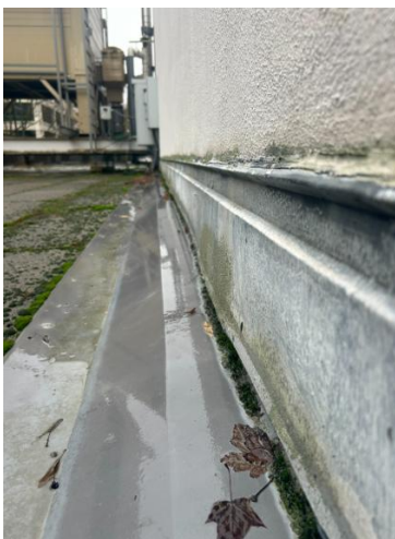
Wear and organic growth observed at wall flashing
