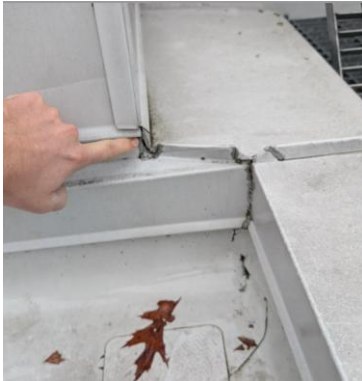
Gap in wall to roof flashing
