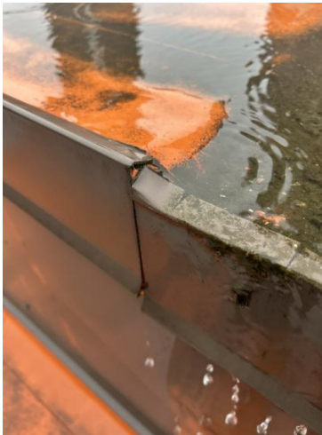
Separation at flashing joint
