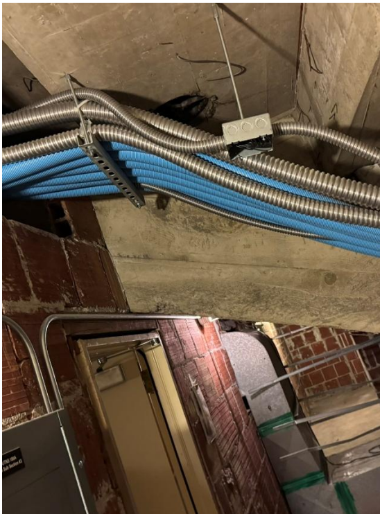
This picture represents typical branch wiring
