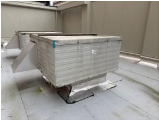
Picture depicts a representative sample. All fans need to be replaced.
